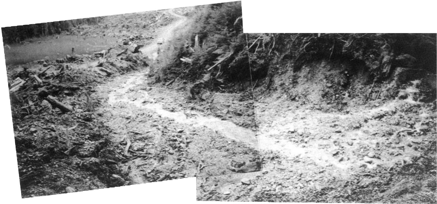
Looking downstream. Deflection berm is on left. Upslope side of berm has not yet been armoured.
