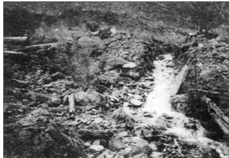
New creek channel on right of photo, old channel on left. Looking upstream from mainline.
